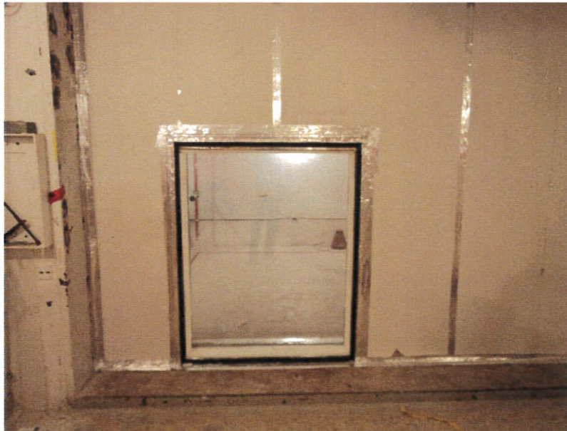
Figure 3. 1496 mm high x 1196 mm wide Magnetite Framing System was installed 100 mm away from the 1418 mm high x 1138 mm wide single pane wood window.
