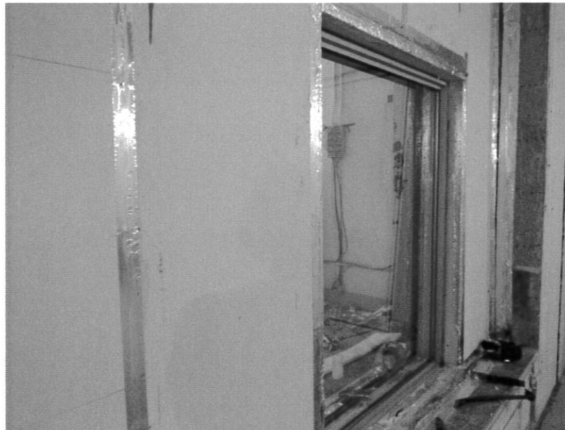
Figure 4. 1457 mm high x 1178 mm wide double pane aluminum window was mounted in the 2440 mm high x 3658 mm wide filler wall.
